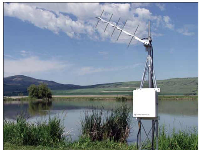
Our GOES transmitters are used for stream stage (shown), water quality, and rainfall applications.
